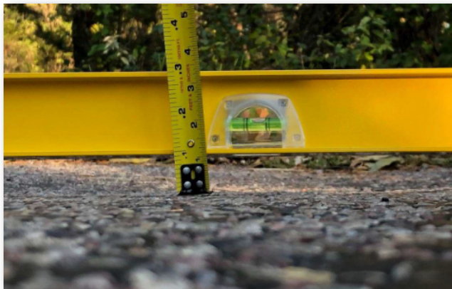
Most Village streets were constructed in the 1950s and now have many transverse dips, cracks and potholes.
